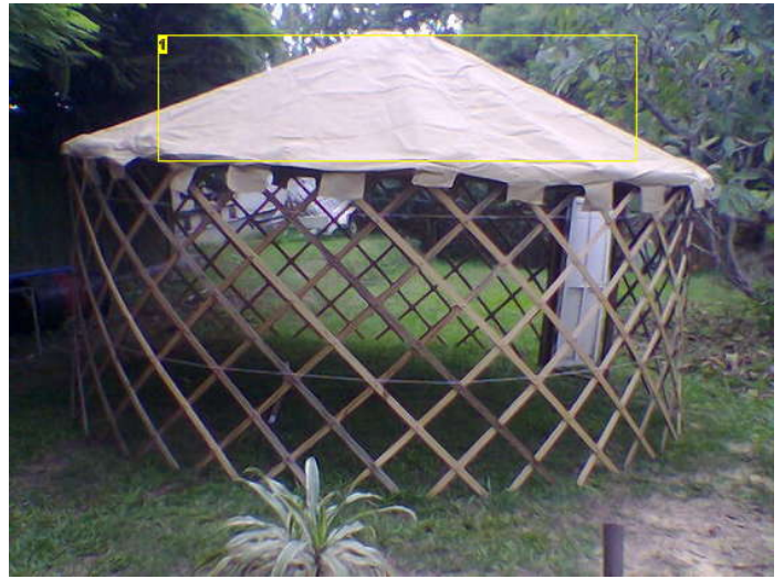
Image Notes 1. loosely fitted roof canvas. (outside view). still a bit crumpled, but this comes out quickly.
